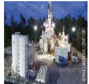
image Geo-thermal research drilling in the Schorfheide done by the Geoforschungszentrum Potsdam, Germany.
